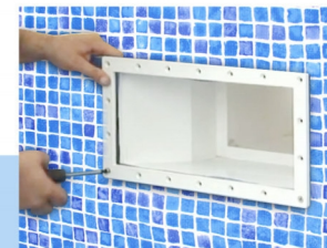
8. 泳池功能件安装 (水口、水下灯等) Installation of hydraulic accessories (water inlet/outlet, lights, etc.)
